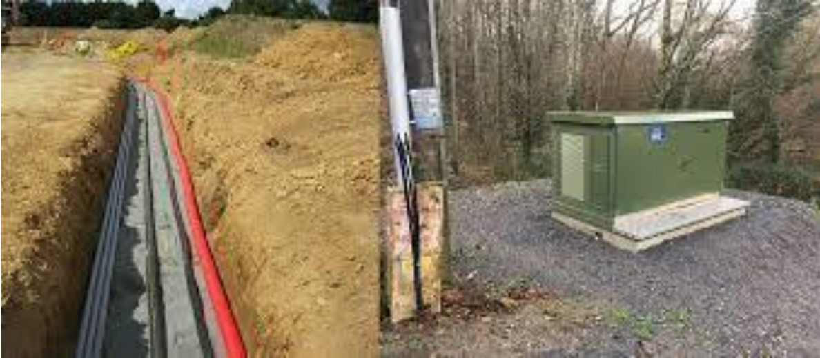
Figure I. 5 : Câble HTA souterrain.
