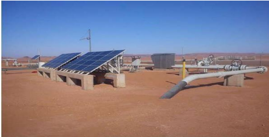
Figure (I.1): Installation photovoltaïque.
