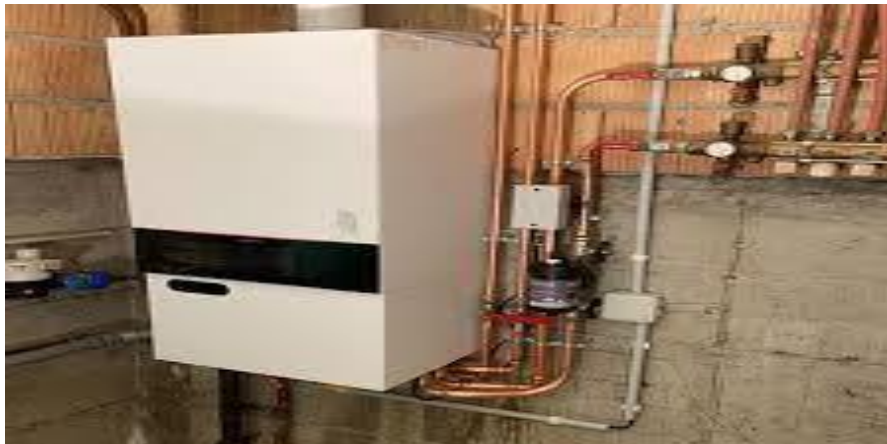
:Figure II-5: Chaudières murales
