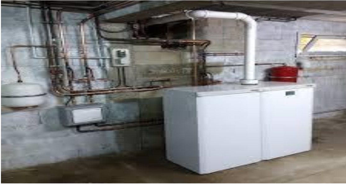
Figure II.4: Chaudières au sol
